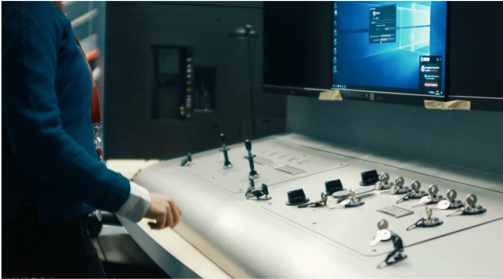
View of the control console integrated into the multimodal EVOC platform- ©CEA
