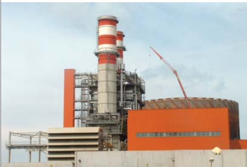
Unit 1 of the new Dunkerque 6 combined-cycle power station French gas utility GDF is planning to put on stream in 2005, close to the Arcelor steel plant. This is the first large gas-turbine, combined-cycle installation to be built in France, with an electricity generation capacity of 2 x 400 MWe.
