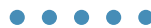
The Purex process, used to recover uranium and plutonium from spent fuel, can also be adjusted to extract iodine, technetium, and neptunium. Shown here are pulsed columns in the T2 high-activity extraction unit at Cogema's UP3 waste-reprocessing plant at La Hague.
