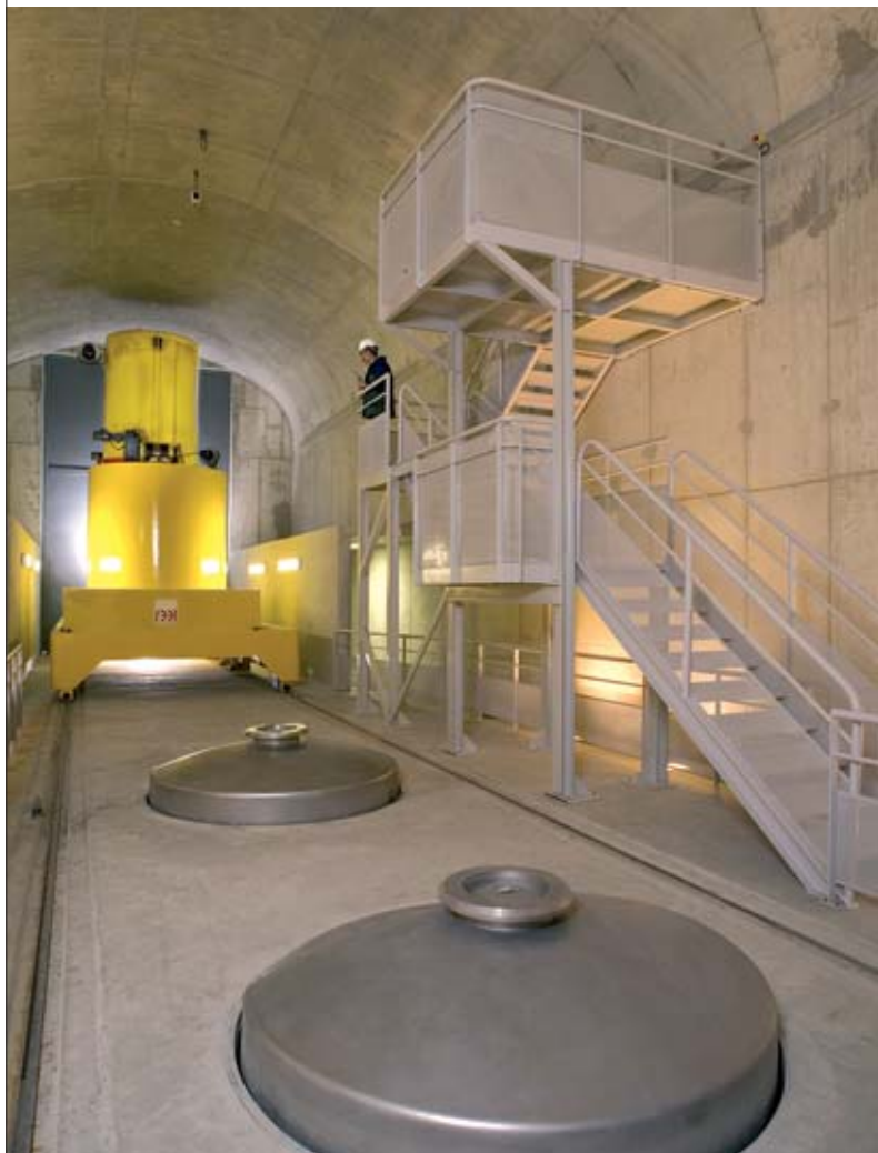
Storage Test Activity Gallery (Galatée: Galerie activités de tests pour l'entreposage ), constructed at CEA's Marcoule (Gard département, Southern France) Center, for investigation of the long-term storage of heat-generating waste. Two well heads and a 170-tonne transfer cask, for container handling, may be seen, in the foreground and at the back, respectively.
