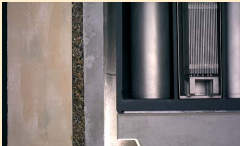
Cross-section of an experimental storage borehole for a spent fuel container (the lower part of the assembly may be seen, top right), in the Galatée gallery of CECER (Centre d'expertise sur le conditionnement et l'entreposage des matières radioactives: Radioactive Materials Conditioning and Storage Expertise Center), at CEA's Marcoule Center, showing the nested canisters.
