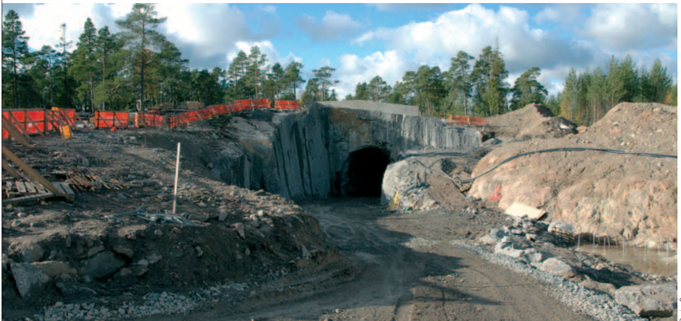
Excavation work for a gallery on the site of the ONKALO underground characterization laboratory, Olkiluoto (Finland).
