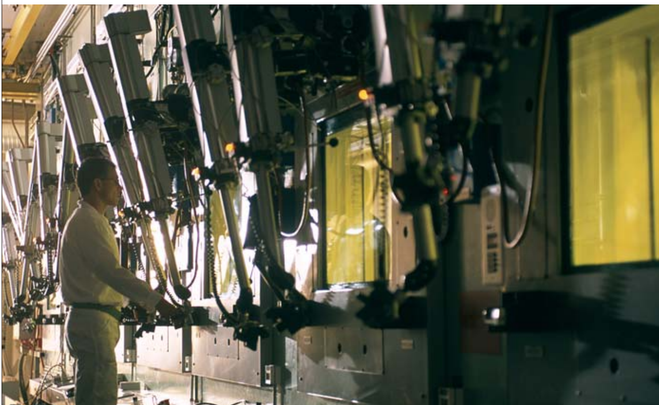
The shielded process line (CBP: Chaîne blindée procédé ) in Atalante, used for the demonstration trials of minor actinide separation processes.
