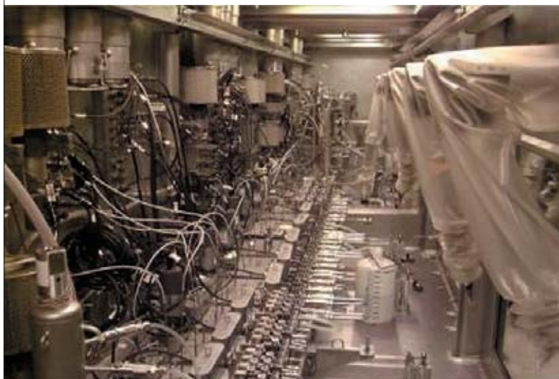
Extraction equipment in the shielded process line (CBP).
