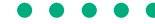
Preparing for hydraulic testing of the vessel (at right) intended for EDF's Civaux 1 power station, at Framatome-ANP's Chalon-Saint-Marcel plant (Saône-et-Loire département, central France). At left, the vessel cover, with control-rod crossings.
