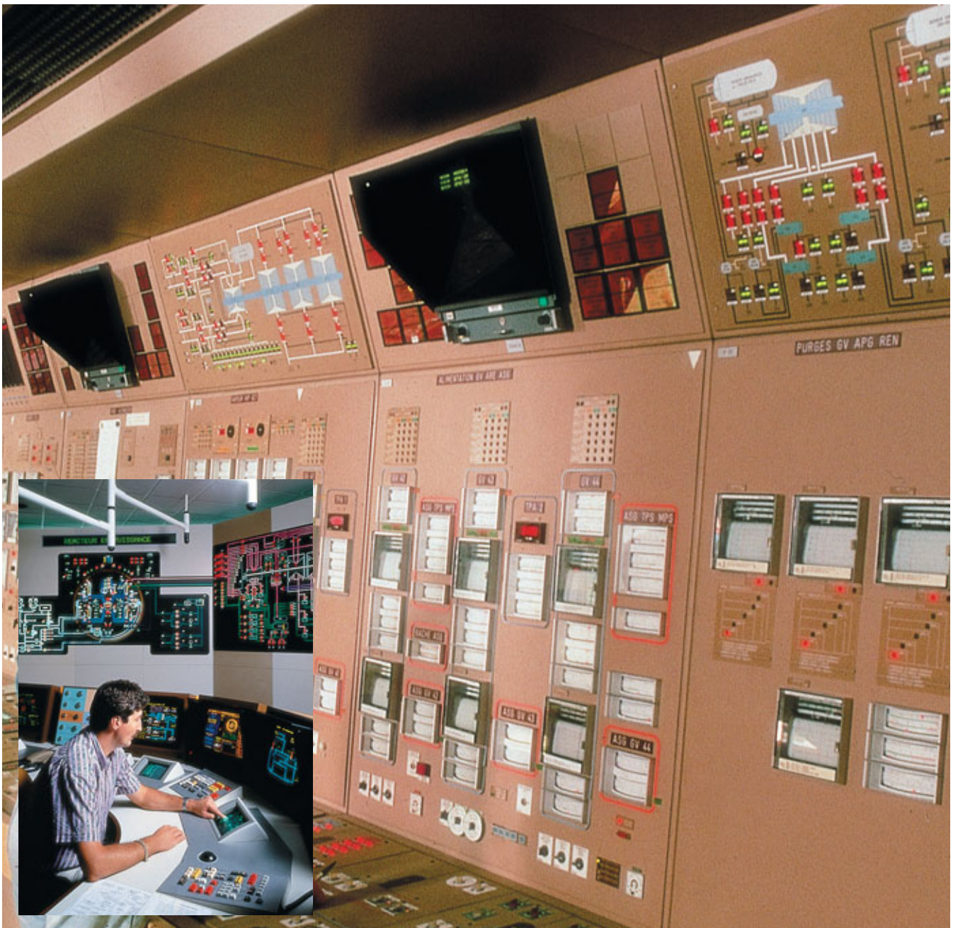
R. de Seynes /P. Berenger/EDF photo library.
