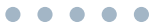
Equipment in the T0 dry unloading shop cell at the Cogema UP3 fuel reprocessing plant at La Hague.
