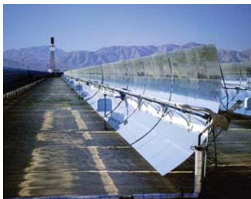
One of the three cylindrical-parabolic-collector solar thermodynamic facilities constructed in the 1980s by Luz Solar in California.
