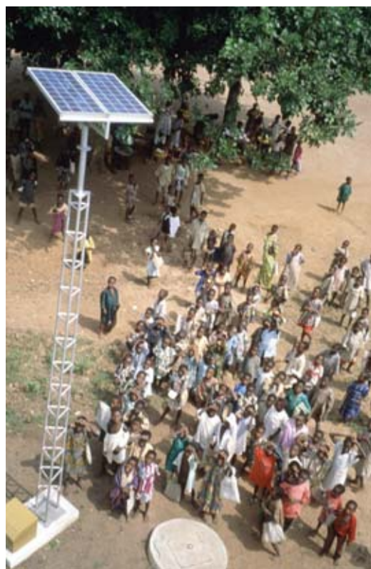
Two solar panels provide part of the power supply for the village of Towé, Benin.
