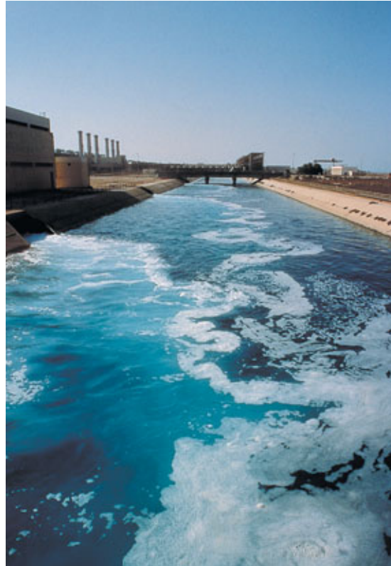
Sea water desalination factory at Jubail (Saudi Arabia). Today, the largest fresh water producers are in the Middle East.
