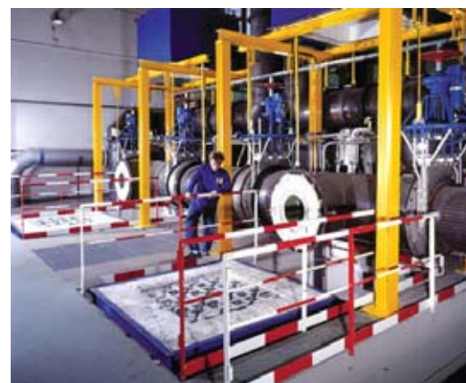
Experimental installation with two regenerators of 5-m height, enabling investigation of thermal behavior of cruciform components, thus allowing optimization of stack configurations.
