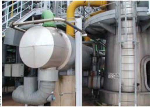
High-performance horizontal-tube heat exchanger, installed at the Knapsack polypropylene production plant, in Germany. The exchanger is positioned at the base of a distillation column, used for polypropylene purification, the base of the column being charged with propane, which is vaporized in the exchanger.
