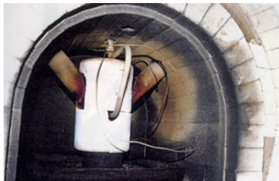
View of the incineration-gas treatment system in the furnace of the MAP plasma waste-vitrification model. This model is set up in the Chicade facility at CEA/Cadarache, and designed for the study of beta-gamma radionuclide distribution between the vitrified product and gas emissions, when waste is processed by plasma melting under conditions representative of real industrial conditions.
