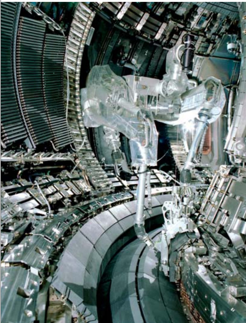
Maintenance robot for the more exposed components of the JET inner wall. ITER will require extensive use of remote handling, particularly for diagnostic maintenance.
