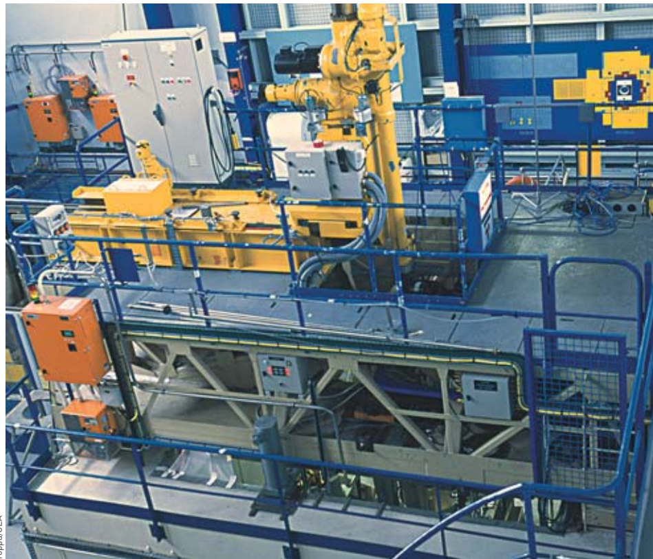
The MINERVE reactor in its hall, at CEA's Cadarache Center.
