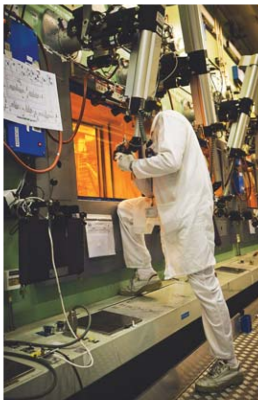
Remote-manipulator work on the shielded process line (CBP) in the CEA Marcoule Center's ATALANTE facility. Demonstration of the technical feasibility of many processes, such as the SANEX, DIAMEX, GANEX and EXAm processes, was carried out on this shielded line.
