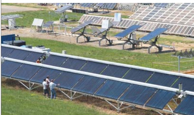
Thermal solar receiver loops in the SAED demonstrator installed on the CEA solar platform in Cadarache. The loops, which measure about 200 m in length and are installed in parallel, consist of all-welded black steel pipes.
