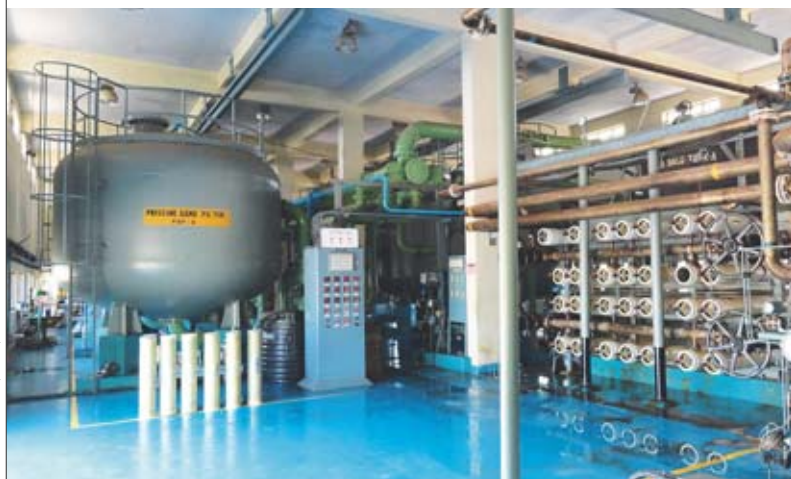
Set of reverse osmosis modules (right) in the nuclear desalination demonstration plant in Kalpakkam, India. The plan comprises a second system based on multi-flash evaporation. These installations, with a production capacity of 6.3 million liters of freshwater per day, are coupled to two Pressurized Heavy-Water Reactors (PHWRs) with a power of 170 MWe each.
