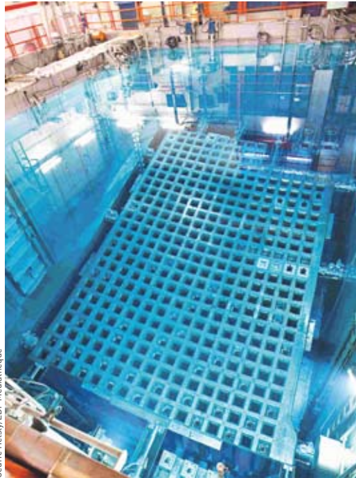
MOX fuel storage pool in the Tricastin NPP (Drôme département). The spent MOX fuels are stored under water in complete safety for reprocessing at a later date. The plutonium they contain, which is in pre-concentrated form, will constitute a resource for the nuclear reactors of the future.
