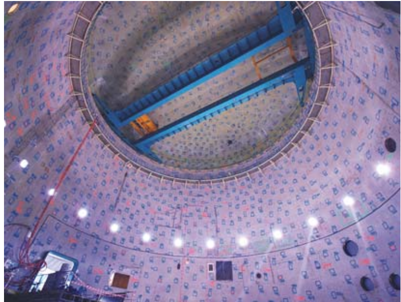
Dome 2 of the Siloé reactor, located in the CEA Grenoble Center, after cleanup and dismantling operations. Radiological checks are carried out on the entire floor and on thousands of points on the walls and ceiling, defined randomly and identified by blue marks.
