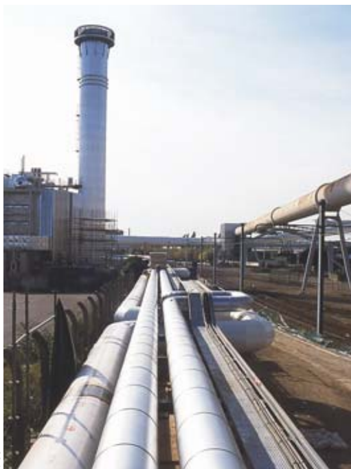
Pipes for heat transport on the cogeneration site of the Compagnie parisienne de chauffage urbain (CPCU) district heating plant at Vitry-sur-Seine (Val-de-Marne département). The site produces both electricity (125 MWe) and steam (400 tons per hour), via a turbine running on natural gas.
